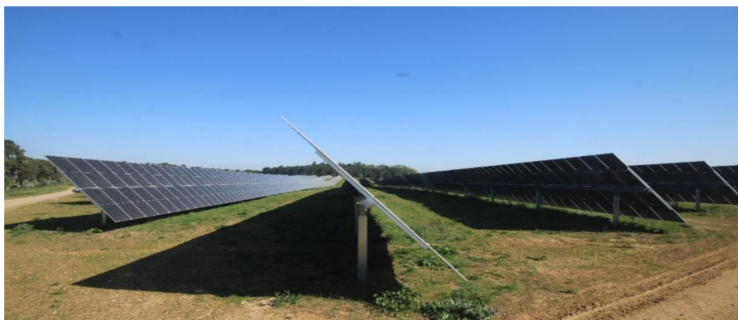
Plate 5-1 Typical tracker Solar PV Panels in an angled orientation
