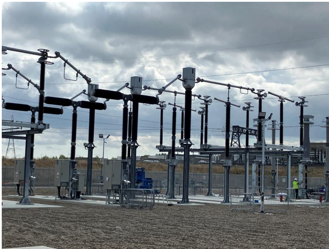
Plate 5-5 Typical 275 kV substation equipment
