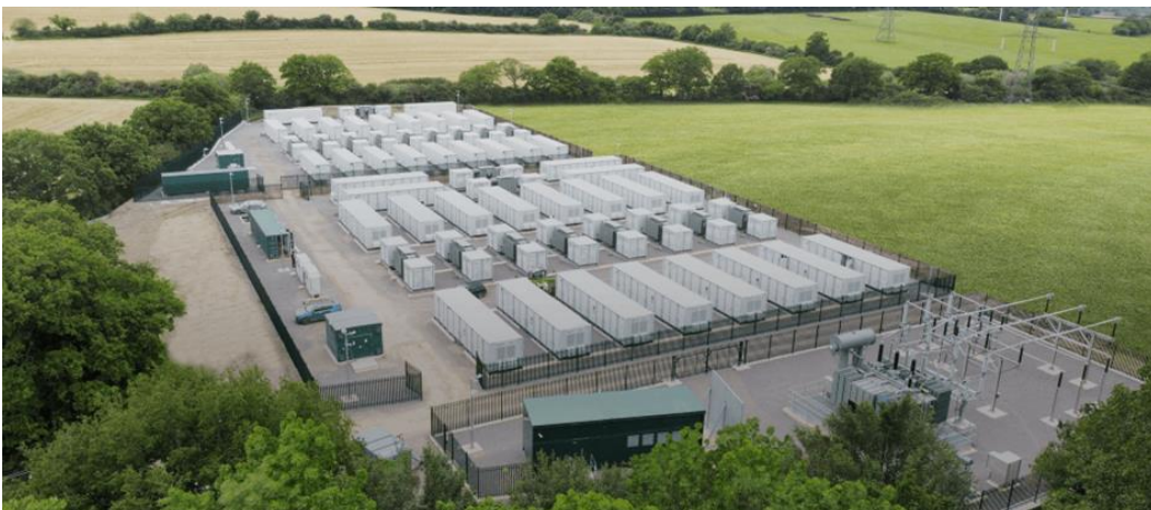
Plate 5-4 Typical Battery Energy Storage System
